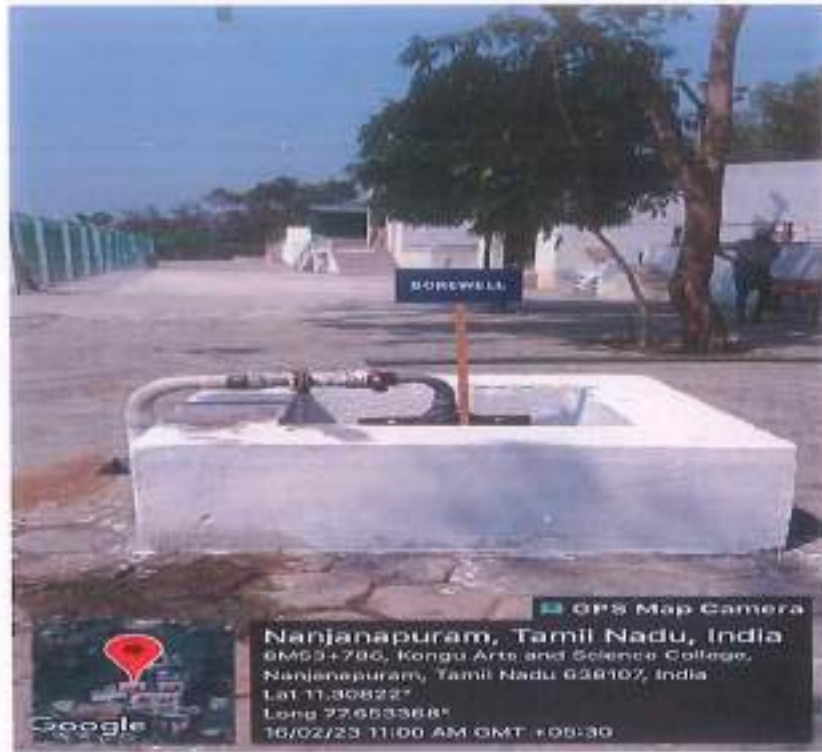
Borewell at STP Plant
