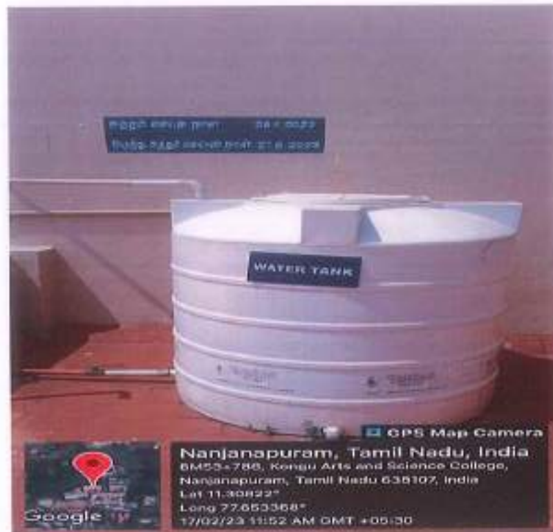
Overhead Mineral Water Tank on the terrace of science block
