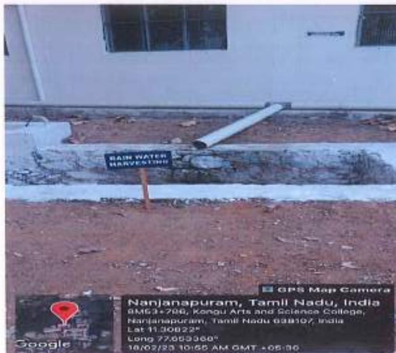
Rainwater Harvesting pit at Library block west side
