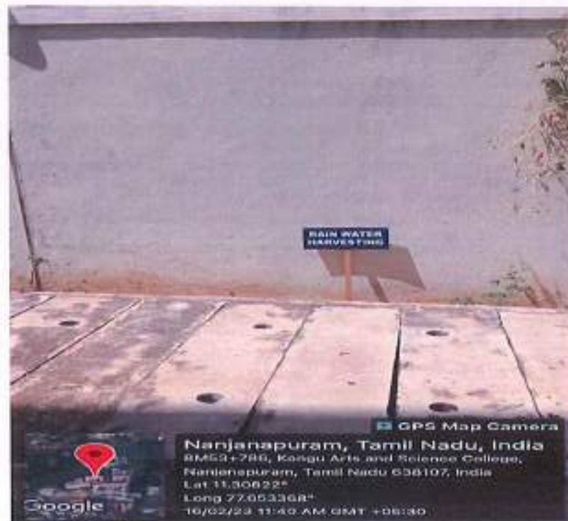
Rainwater Harvesting pit at Staff Quarters
