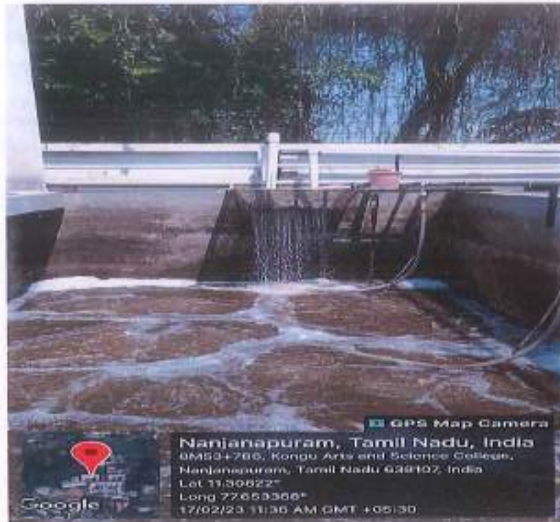
Sewage treatment process at Boys hostel back side
