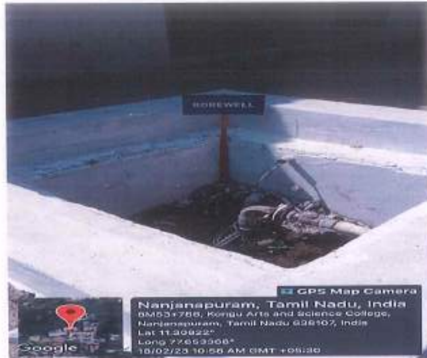
Borewell near at the Open Auditorium
