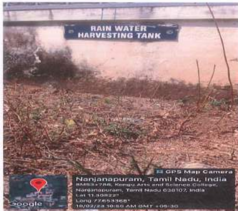
Rainwater Harvesting pit at near open well
