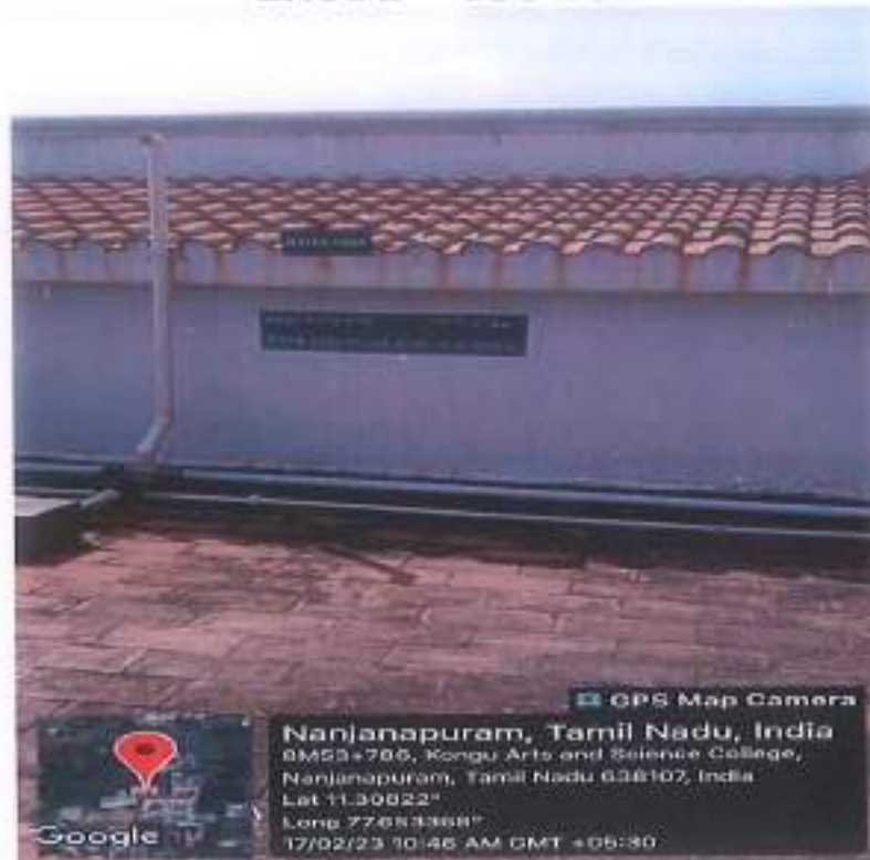
Overhead Ordinary Water Tank on the terrace of main block
