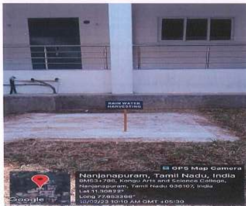
Rainwater Harvesting pit at Stitching Lab back side
