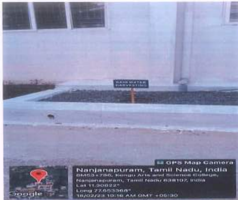
Rainwater Harvesting pit at Main Building back side
