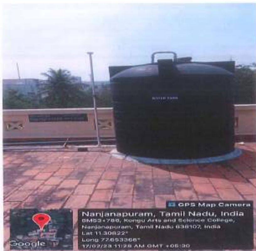
Overhead Mineral Water Tank on the terrace of boys hostel
