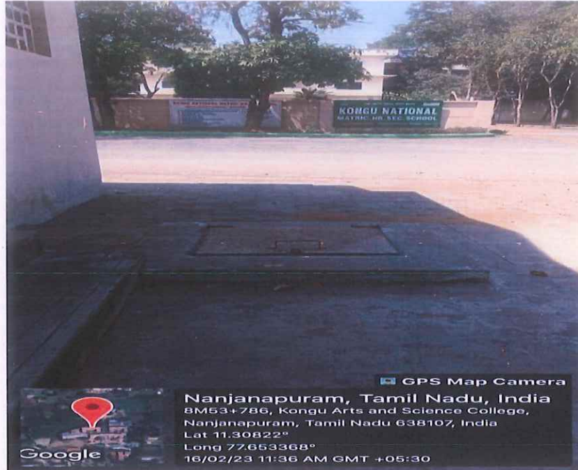
Overall Collection tank near the staff quarters vehicle parking
