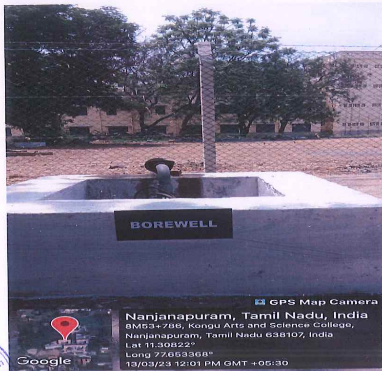
Borewell at STP Plant
