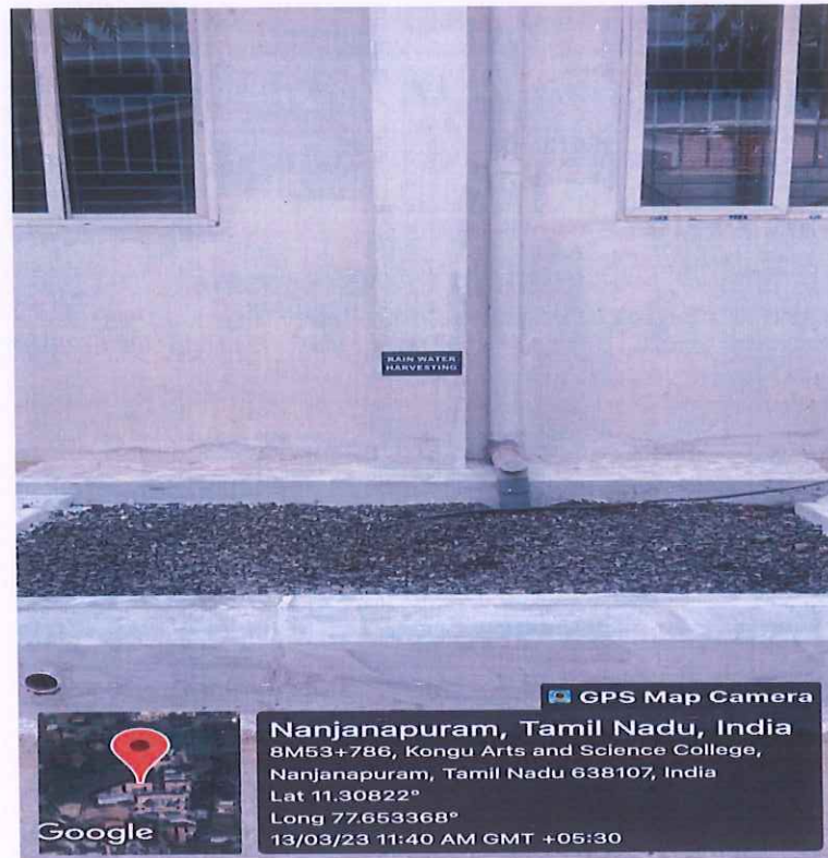
Rainwater Harvesting pit at Main Building back side
