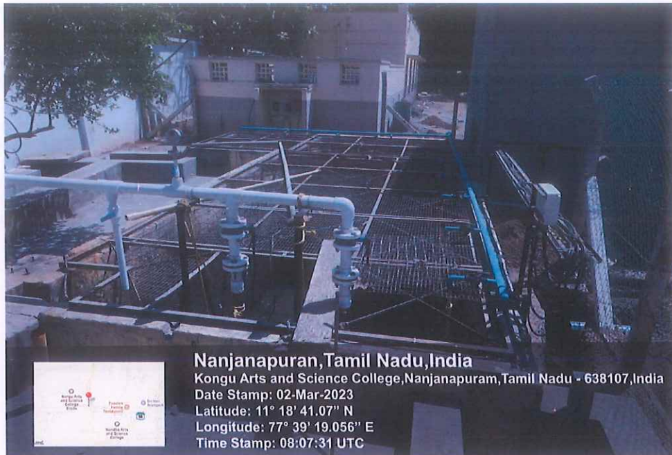
WASTE WATER RECYCLING PLANT
