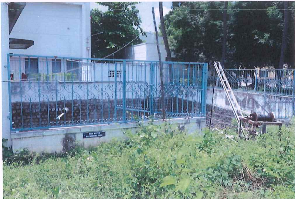
RAIN WATER HARVESTING TANK
