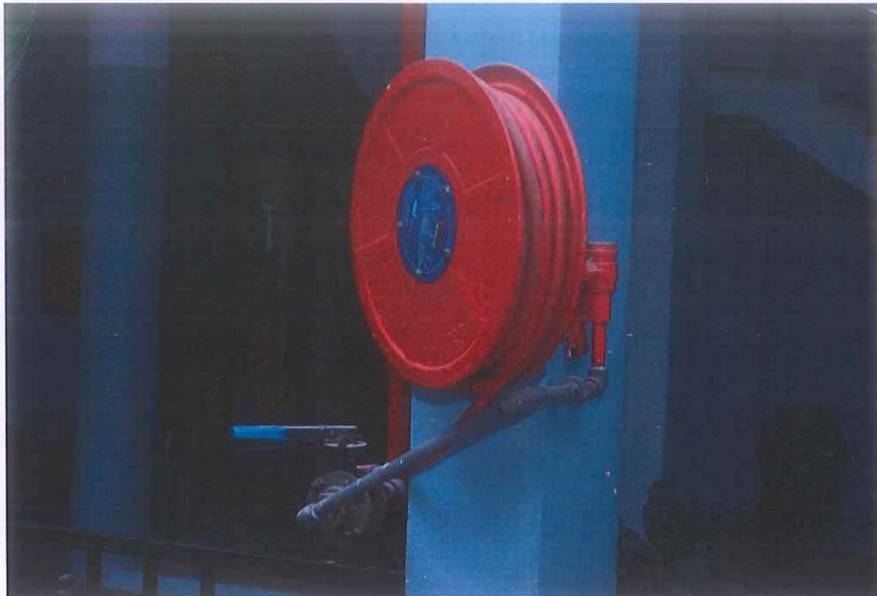
FIRE SAFETY INSTALLED IN BUILDING
