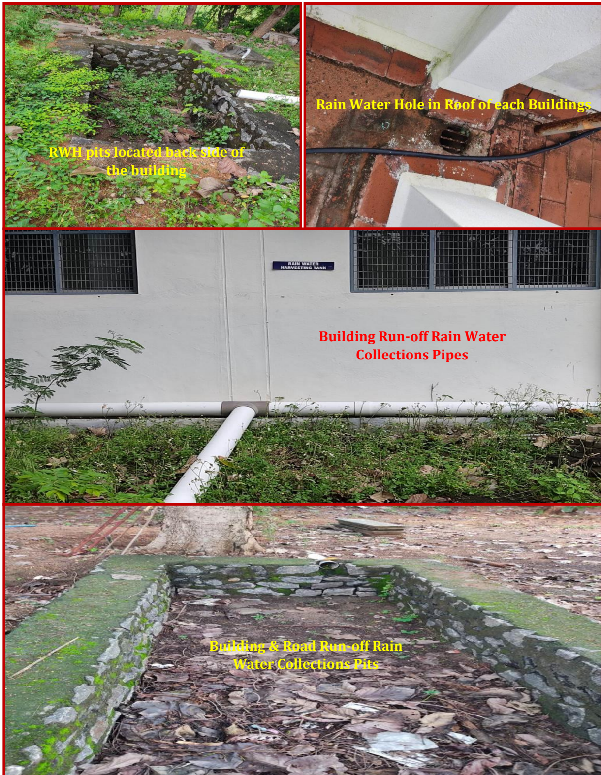
Fig.4: Rain Water Harvesting (RWH) system implemented in the College
